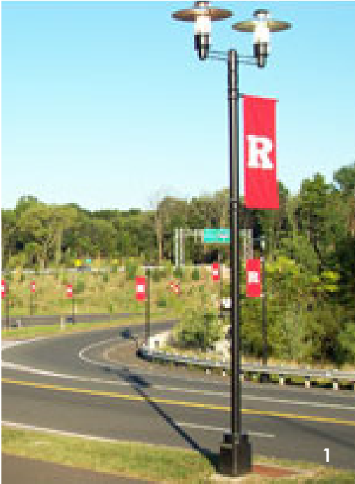
TWO HEAD AREA LIGHTING POLE
