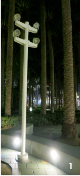
POLE MOUNTED LIGHTS
