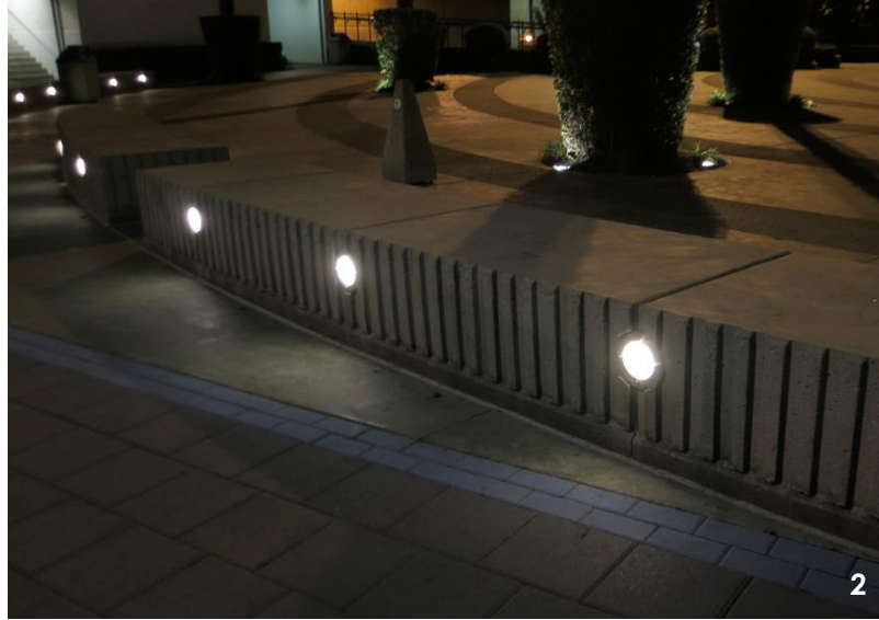
LOW LEVEL PATHWAY LIGHTS
